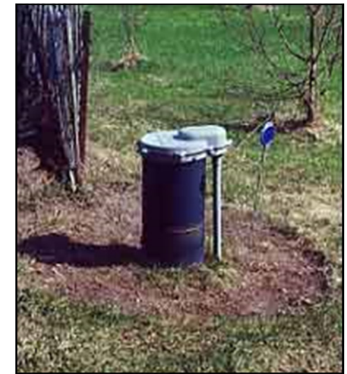
Having a firmly sealed cap and keeping the area around a well free of landscaping are two of the best ways to limit the possibility of bacterial contamination from insects and animals.
